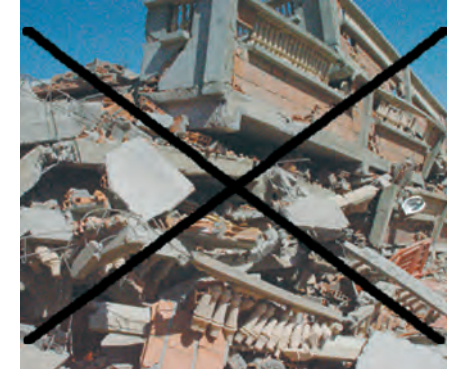
Shear walls would have avoided this earthquake damage...
